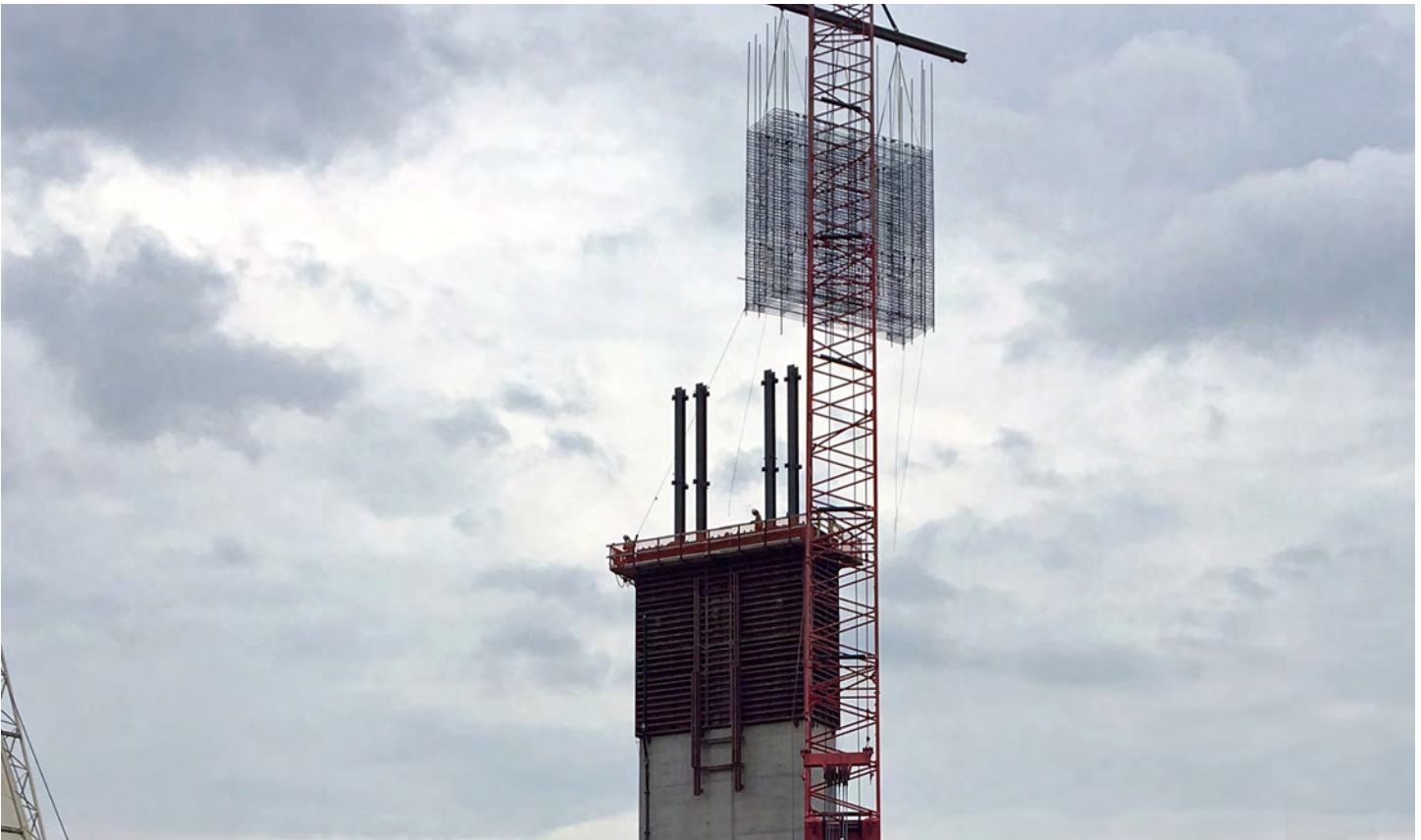
Mechanical couplers being lifted into place for a pier stem. More than 10,000 mechanical couplers were used to join the steel reinforcement within the various concrete portions of the river bridge.
