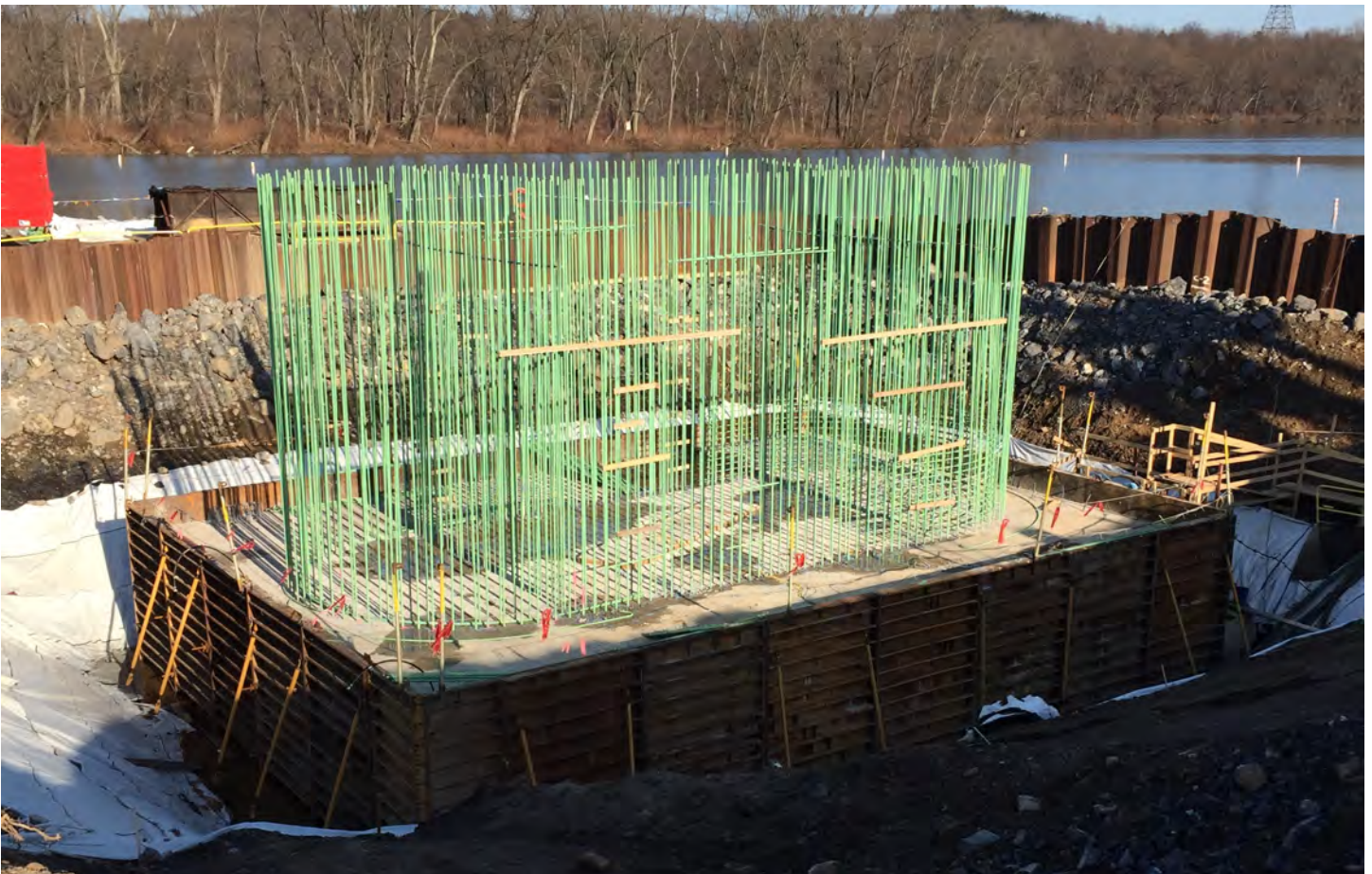
A river pier foundation with 1,000 cubic yards of concrete and initial steel reinforcement for the pier stem in place.
