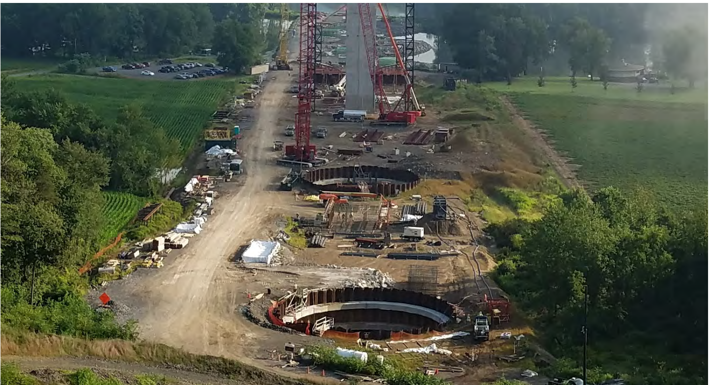
Circular temporary excavation support (shoring) systems used to construct several land pier foundations. A completed pier stem is also visible in the background.
