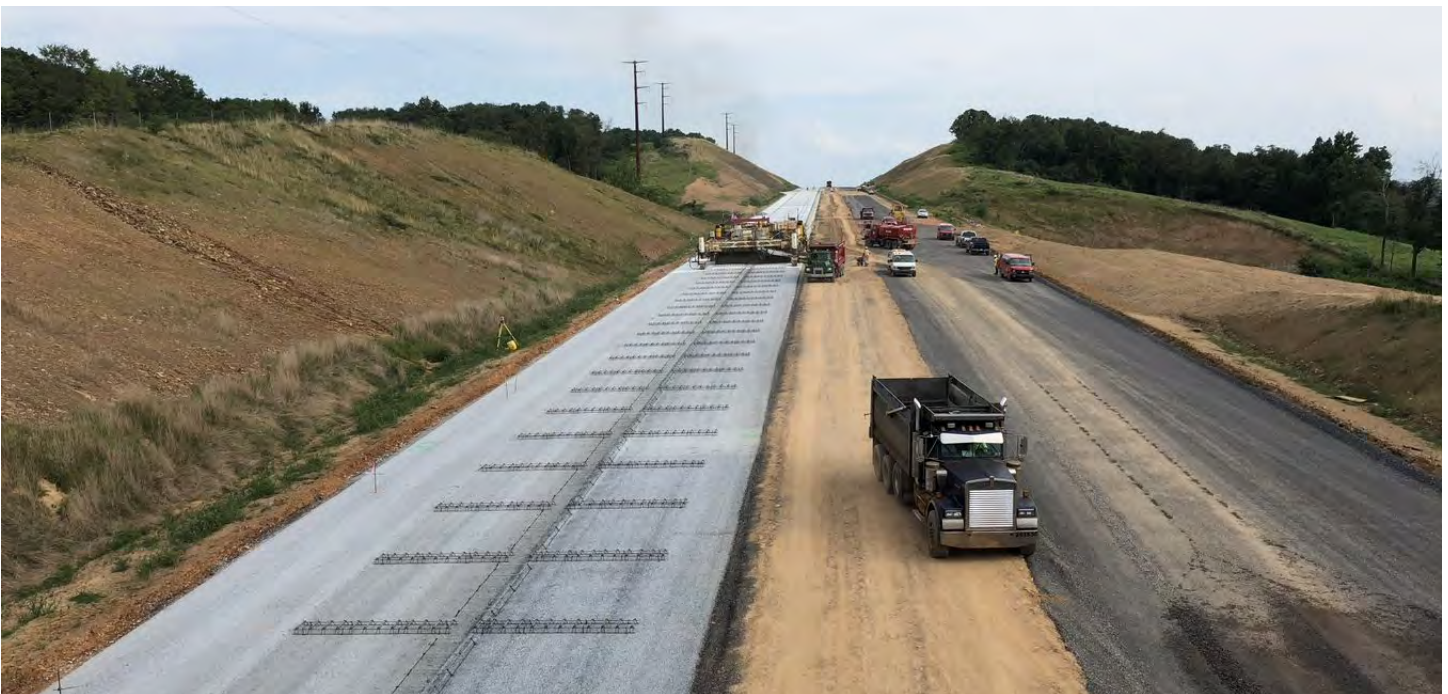
Construction of the highway pavement. Shown on the right is the subbase course consisting of 2A aggregate, and shown on the left is the cement-treated permeable base course placed on top of the subbase, prior to the placement of concrete pavement.
