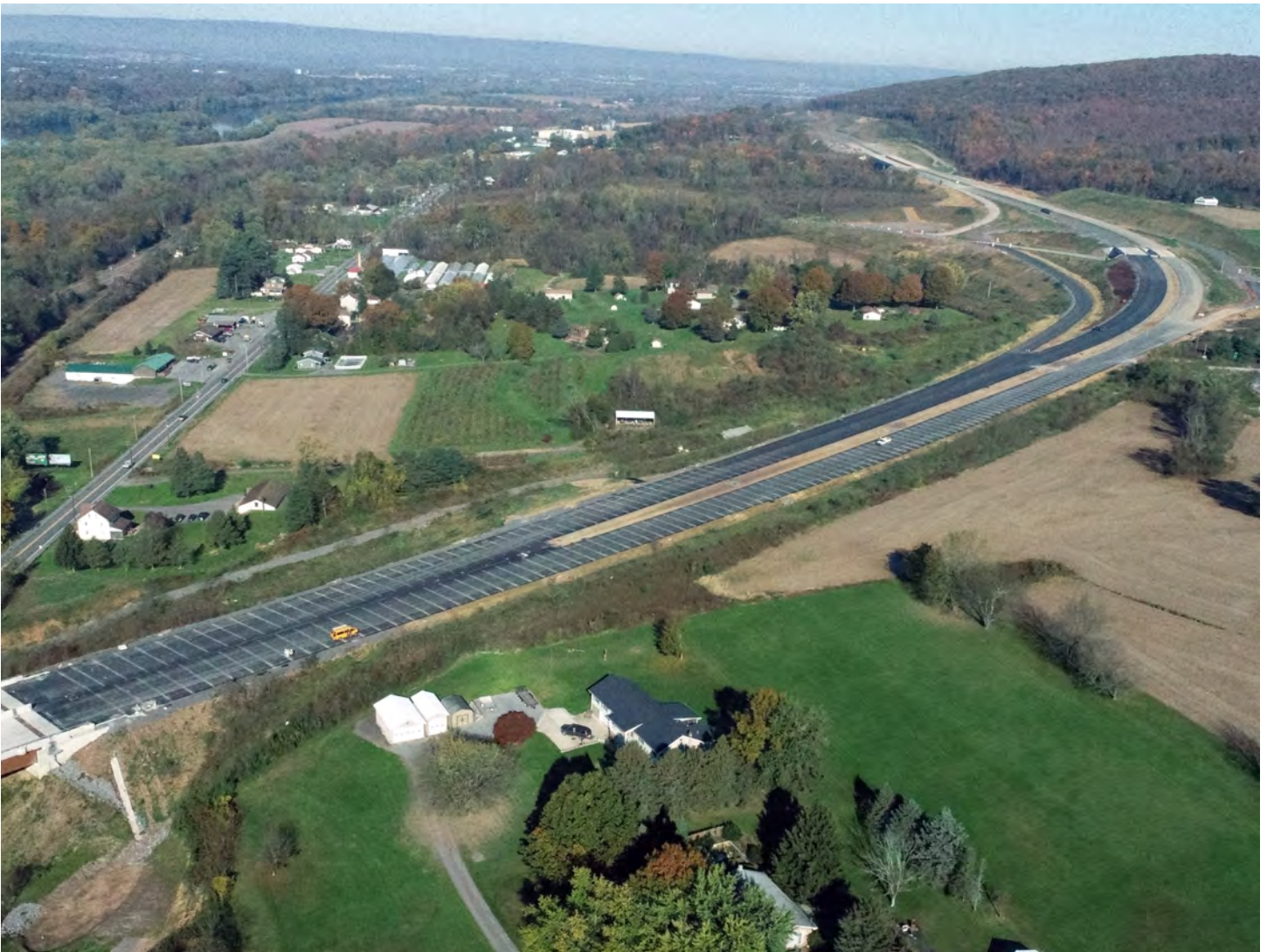
The intermediate asphalt layer (binder course) placed on top of the concrete pavement, looking north from the north end of the river bridge in Northumberland County.
