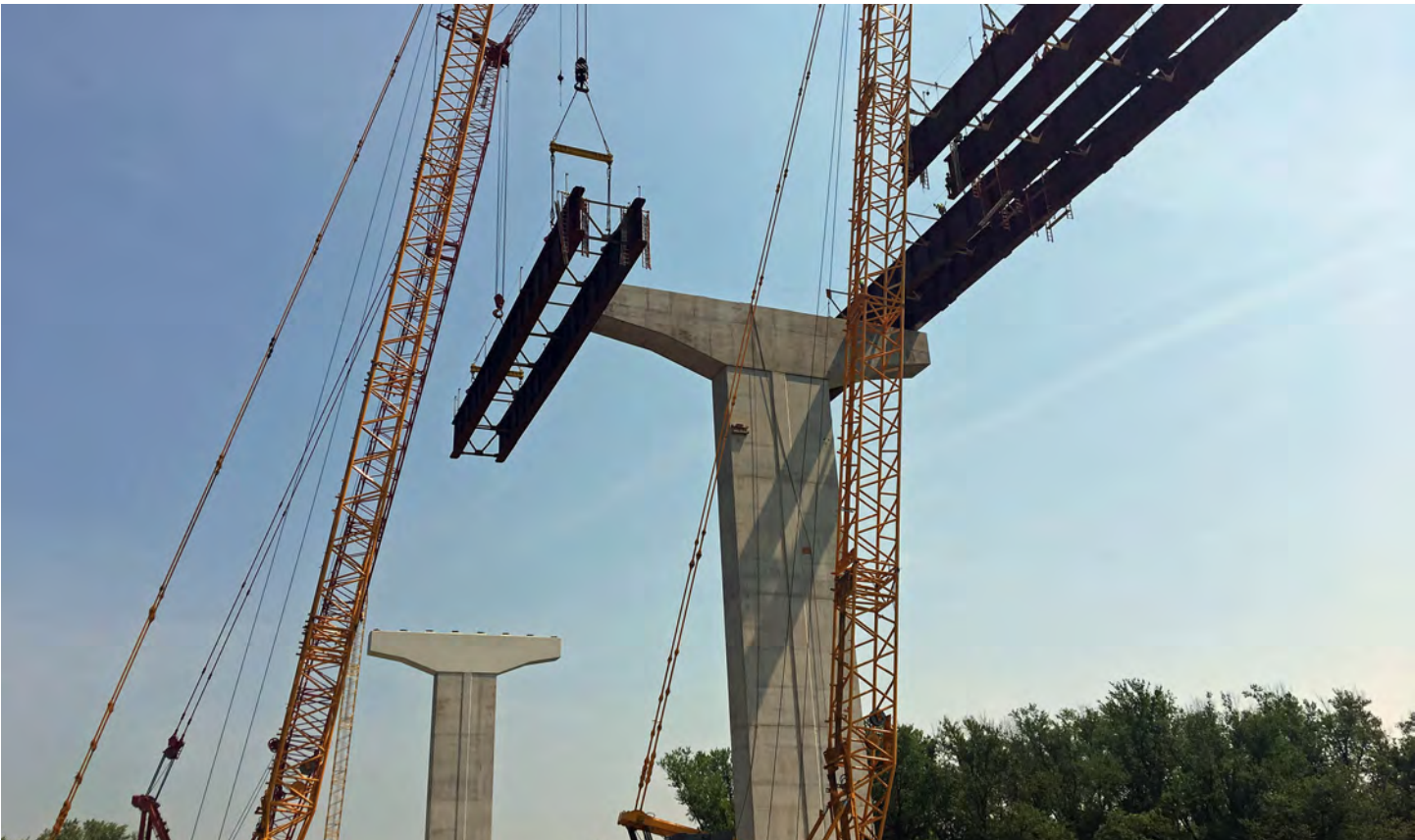
The first beams being set in place. The beams are 10-foot-high steel I-beams.
