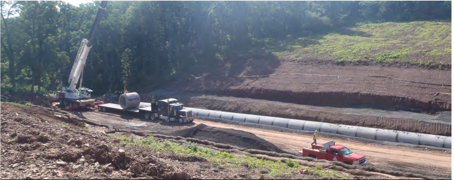
An 84-inch diameter concrete stream culvert located south of County Line Road at the southern end of the CSVT Northern Section.
