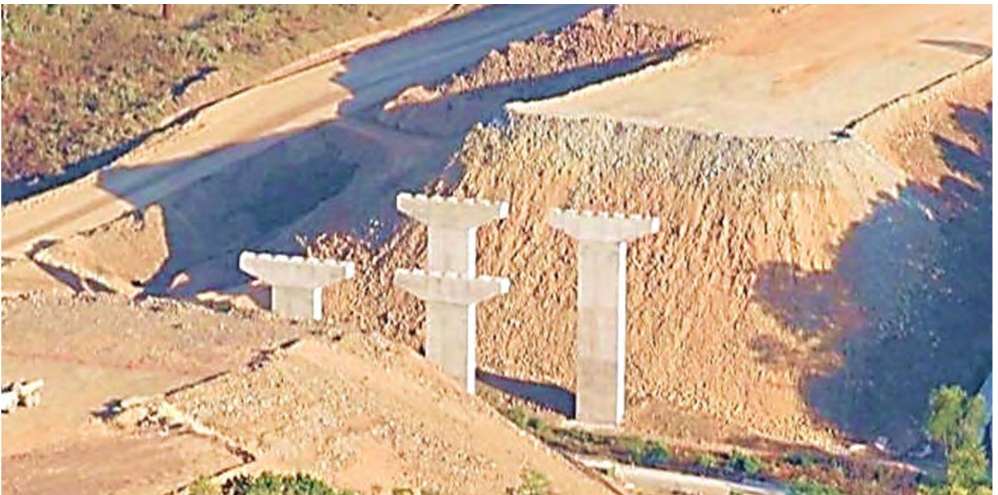
Completed piers for the bridges over Wooded Run and Hollow Road. The embankments shown were constructed and then quarantined and monitored for settlement prior to constructing the bridge abutments.
