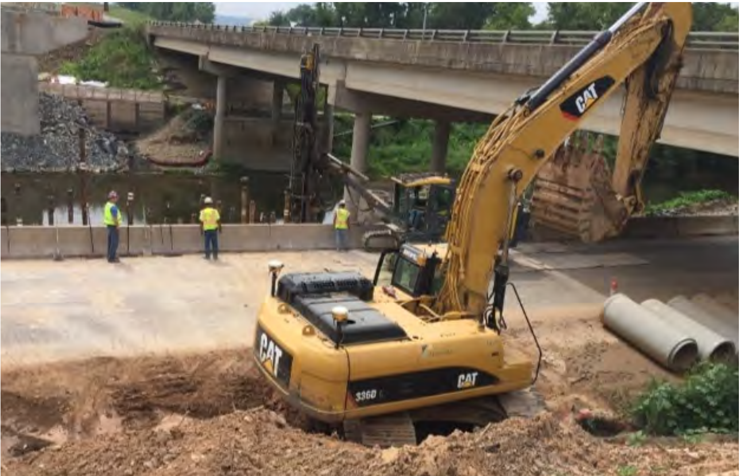
Construction of the new 3-span bridge over Chillisquaque Creek (on the left) and the existing bridge that was later removed and replaced (on the right).
